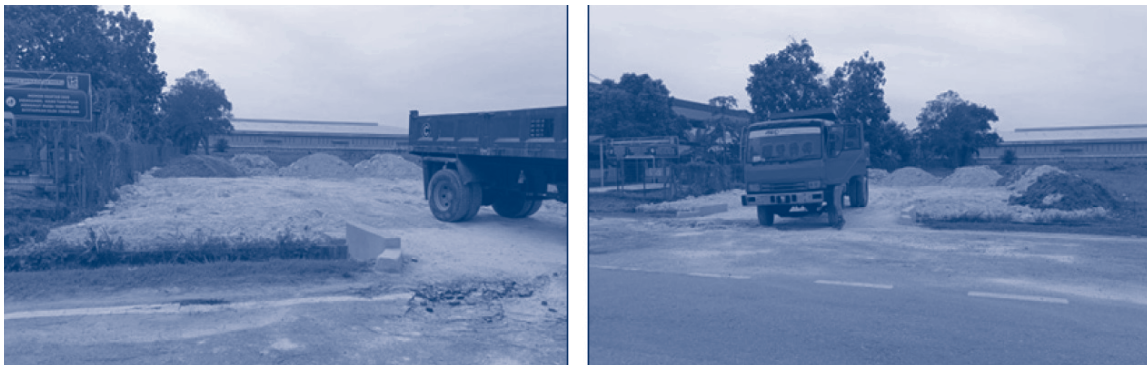
Figure 4.2.1 Lorries transporting red soil to Sekolah Kebangsaan Meru, supporting the development of a new parking area to enhance safety and ease traffic congestion.
